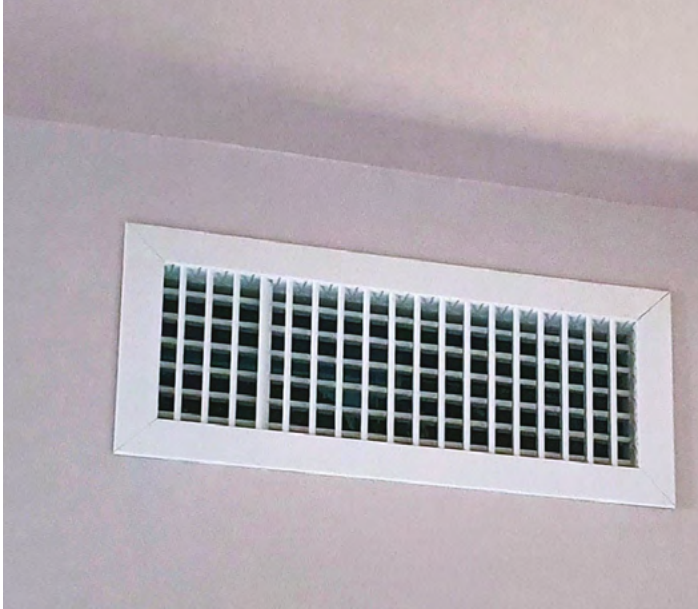
BMA Installation of double deflection nozzle.
